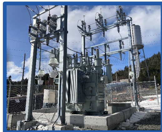
Tors Cove Substation Transformer.
