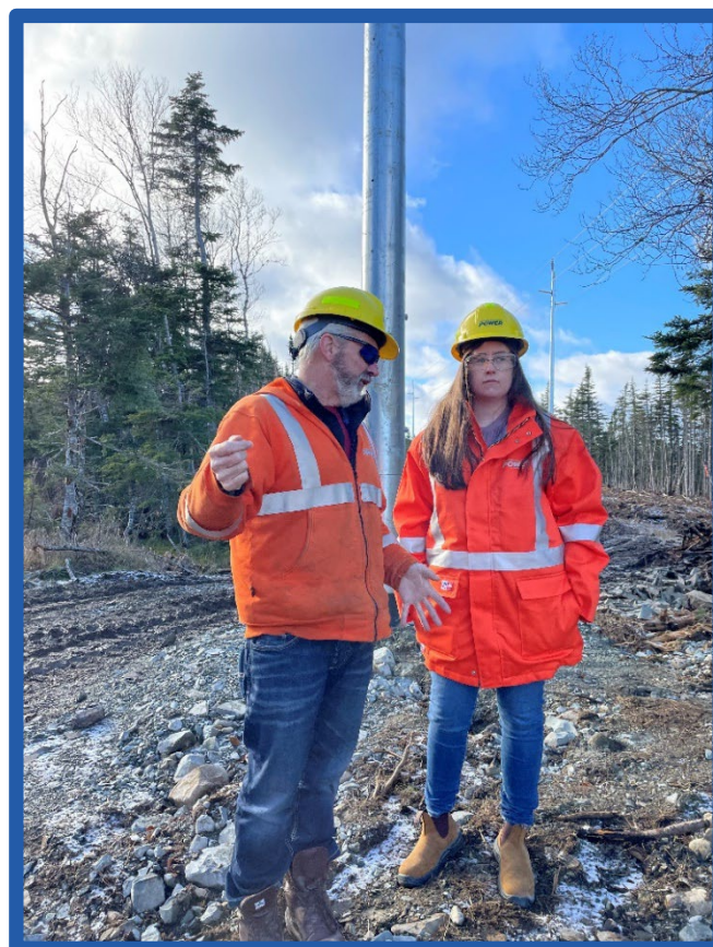
Transmission Line 35L in St. John's area.
